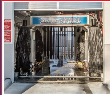
At the Ford Site, AUTEC's system is installed in a bay where hand washing had previously been done.
